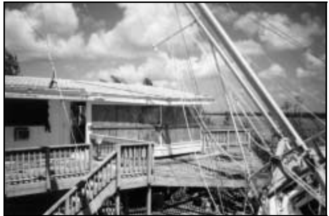
Jack Clark's residence at Ramrod Key, Florida after hurricane Georges seriously damaged it in 1999 and washed a 55 ton schooner into his front yard. Photo courtesy of Don Clark
